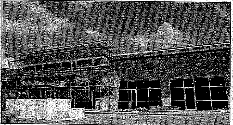
The new Highlands Plaza development off of Loop 336 is nearing completion. Workers installed the glass shop windows in Highlands Plaza's shopping center Tuesday. Staff photo by Eric S. Swift.
